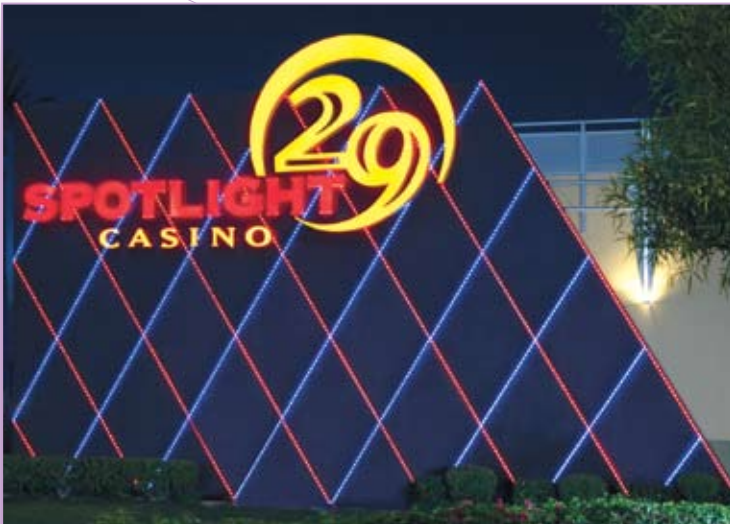
LEDs installed in Trillium Channel provide a perfectly linear effect of color-changing light.
